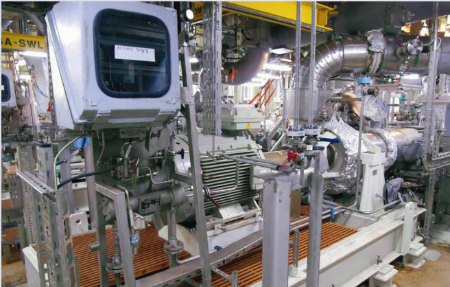
Finder crude oil transfer pump sealed with H75FD/90-E3-A1 dual seals, supply in accordance with API Plan 53B.
