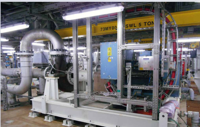
Finder cooling medium circulation pump sealed with single seal H75VN/90-E88-A1-OR, supplied in accordance with API Plan 11.
